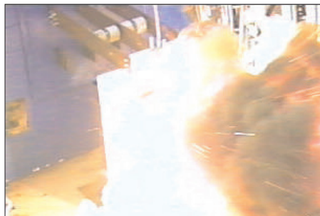
Arc Flash in test lab. Test conditions: 480V; 47,700A; 0.1 second clearing. Incident energy was measured to be 14.9 cal/cm 2 at 18 inches.
